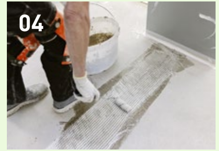
Insert corrugated connectors into the cuts and seal with resin. Then apply fibreglass fabric and sand with quartz sand.
