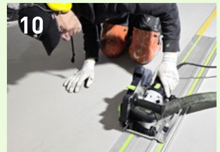
Cut open any filled-in expansion joints with the DSC AG 125 and a guide rail. Tip: For longer expansion joints, several guide rails can be connected.
