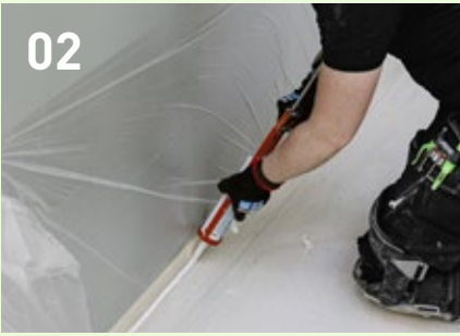
Use acrylic sealant to fill the joints between the edge insulation strips and the floor.
